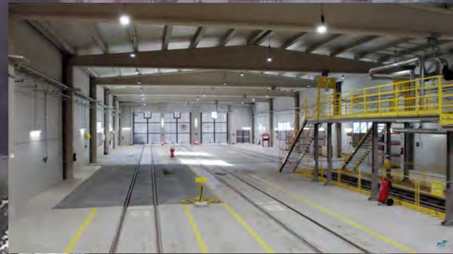
Interior of the new building installed at Benidorm station, which will allow trains to be stored, serviced and cleaned.
